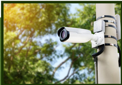
One Gate System & CCTV 24 jam
